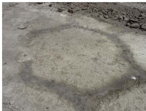
Figure 7. The photograph was taken by an unidentified engineer working on a new subdivision in Saskatoon. It illustrates the polygonal pattern of dark, organic matter-enriched topsoil that has fallen down cracks in a Vertisolic soil, probably at a depth of 50 to 80 cm, and exposed as surface soil was excavated. The photo also indicates the need for special practices to deal with the swelling clays, and possible future problems with streets, sidewalks and basements.
